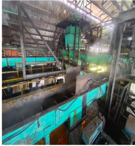
Gambar (a) pembagian distributing conveyor
